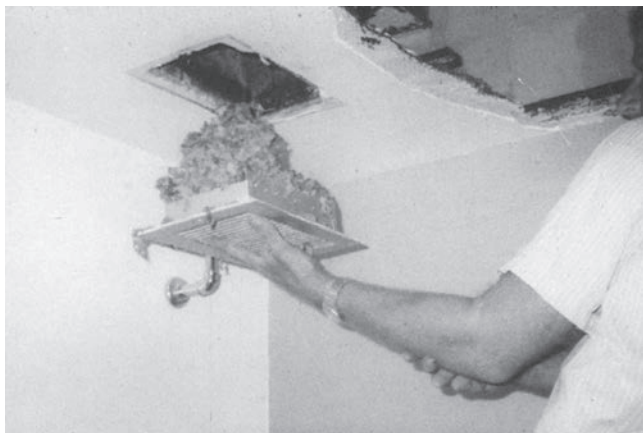
FIGURE 71-3 Bathroom exhaust debris.
